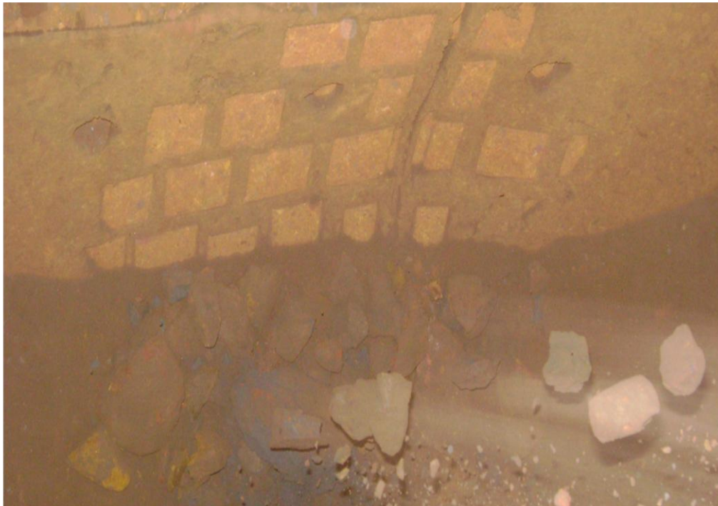
TEGA MOSAIC LINER INSTALLED IN CHUTE HANDLING IRON ORE LUMPS
